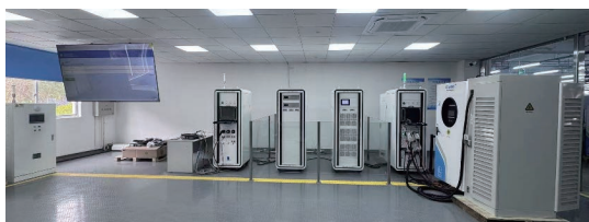
Remote Intelligent Metrology Cabin for EVSE
